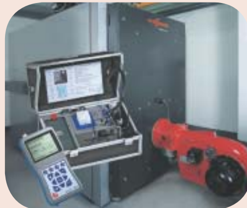
J2KN at Viessmann oil boiler
